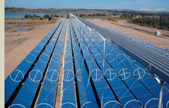
▲ An Ausra plant in New South Wales, Australia. Ausra will use the same technology to construct carbon-free power plants designed to fulfill the commitment made at the Clinton Global Initiative. Their existing plant is at the Liddell Power station, providing high-quality steam to Macquarie Generation, Australia's largest generator. The new commitments announced by the company will lead to the construction of similar plants in the United States.
