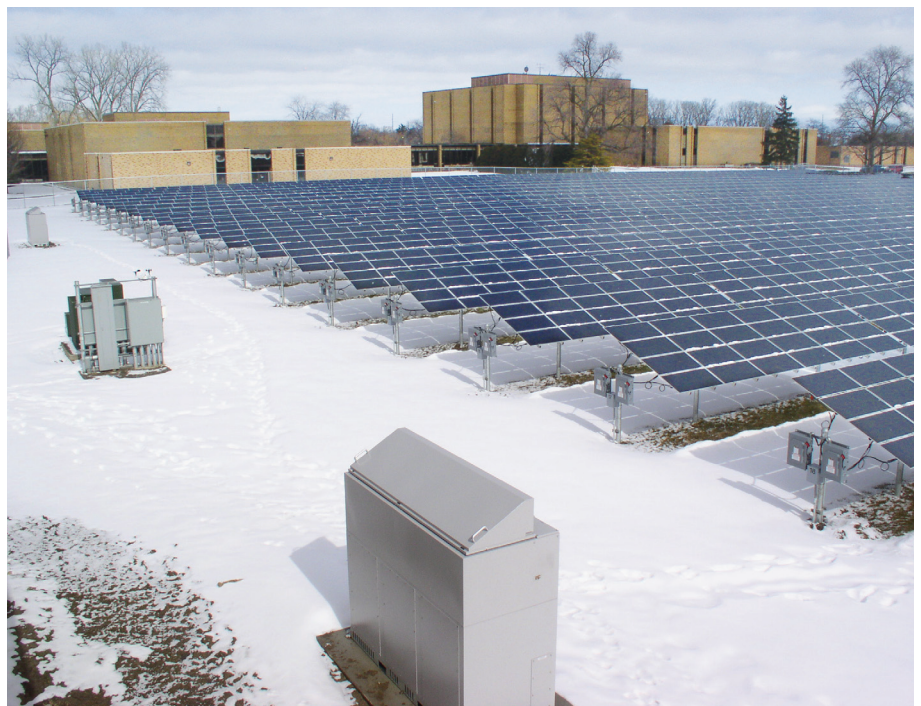
This 1 MW PV installation in Ohio, installed by Advanced Distributed Generation LLC, uses 260 kW PV Powered inverters.
