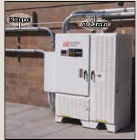
The AE Solaron® 333 kW inverter installed at Cline Cellars
